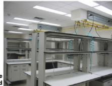
Infrastructure Raceway and
